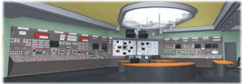
Advanced Digital Control Room - Installed in Qinshan, China Nuclear Power Plant
