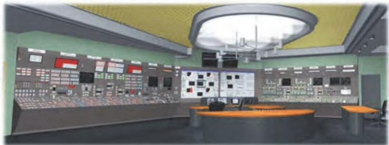
Advanced Digital Control Room - Installed in Qinshan, China Nuclear Power Plant
