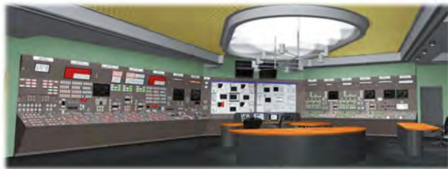
Advanced Digital Control Room - Installed in Qinshan, China Nuclear Power Plant
